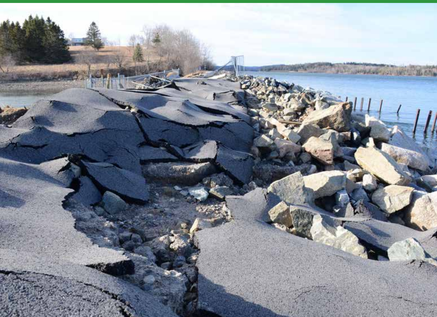
Erosion on a coastal path, St Andrews, New Brunswick
