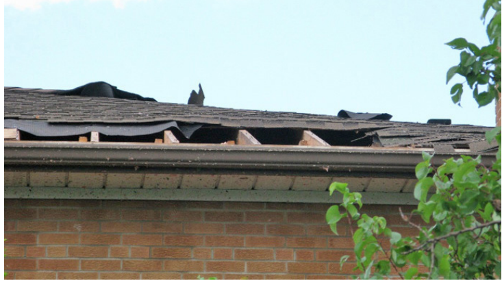
Photos of sheathing loss after wind event (GTA area houses).
