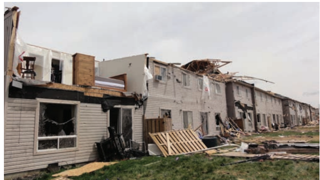
Figure 2: Structural roof failures (Angus, Ontario 2014)
