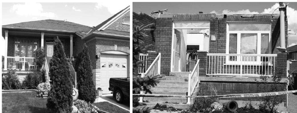
Figure 3: Side-by-side damages – one home with damages consistent with DOD 1 or 2, the next with a global roof failure, consistent with DOD 6 damages 34
