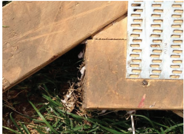
Figure 4: Incorrect roof-to-wall connection (Vaughan, 2009)
