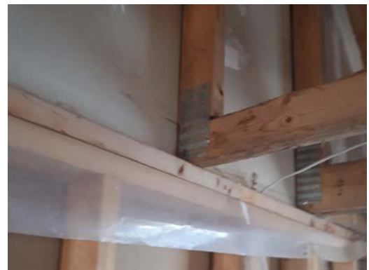
Figure A.3: An example of a roof-to-wall connection where provision of toe-nails is difficult (roof truss, minimum end bearing, southern Ontario)
