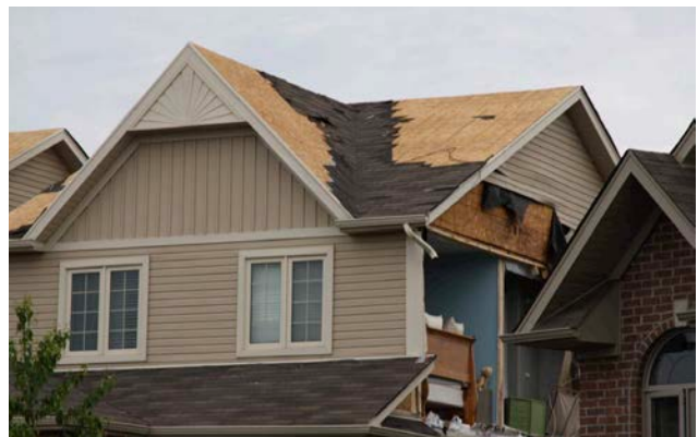
Figure 5: Wall failure indicating issues with construction (Angus, 2014)
